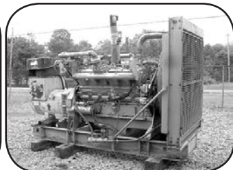
'97 New age Stamford 255 kW , Cum. V12, natural gas powered generator, 3-phase, 208 volts, LESS THAN 1 HR. USE! Half price of new, $12,500.
